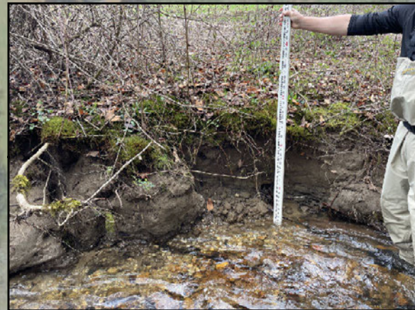
Site 13 (60 linear feet, left bank) Estimated erosion rate: 0.9 tons/year
