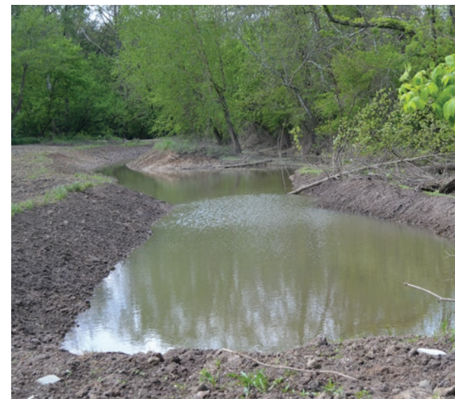
Earth movers have begun digging out three sloughs, including this work-in-progress. Ultimately, the floodplain restoration will benefit fish, ducks, songbirds, turtles, salamanders, insects, mammals and more.
